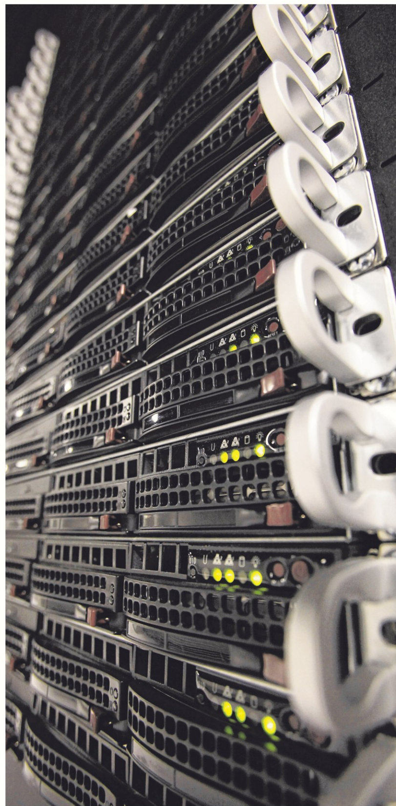
A cloud rack containing servers and hard drives at IBM's Softlayer data centre. Data storage locations will be as essential to daily life as power plants. PHOTO: BLOOMBERG
